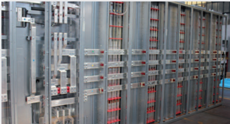
Retro sbarre omnibus e calate verticali Back omnibus busbars and vertical drop
